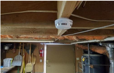
Basement alarm also one in the wood area.
